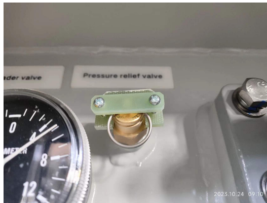
figure 8-19 Pressure Relief valve
