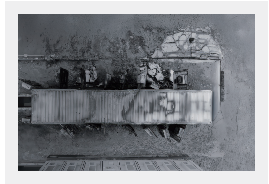
Figure 14: Thermal Runaway Fire Caused by Overcharging Due to 66% SOC Estimation Error at a 20 MWh Energy Storage Station in 2023
