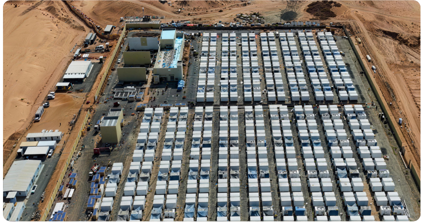
Figure 18: 7.8 GWh Grid-Forming Energy Storage Project in Saudi Arabia
